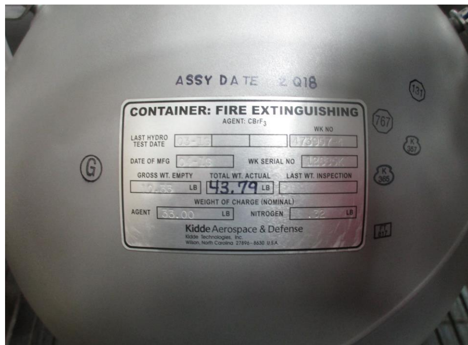
Figure 1: Tested and Refilled Fire Extinguisher
