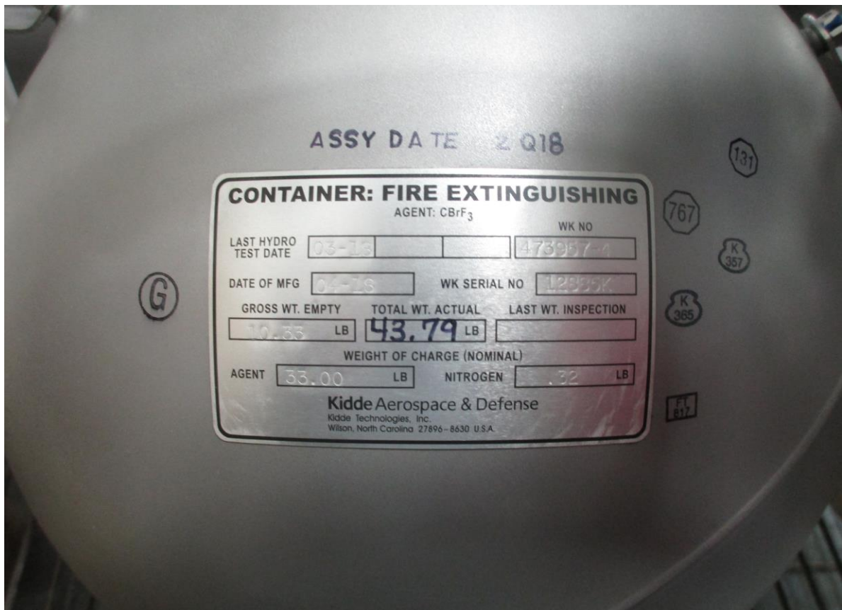
Figure 1: Tested and Refilled Fire Extinguisher
