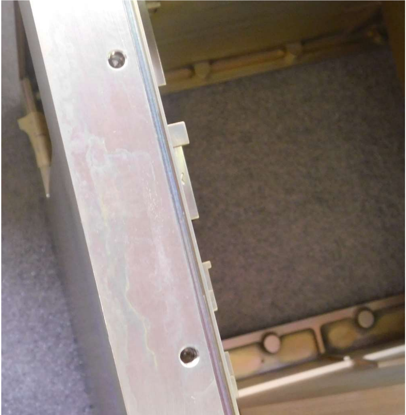
Figure 10: Another example of chemical conversion coating staining.
